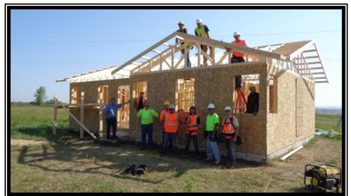
ACC Framing School at Sioux Valley Dakota Nation, near completion of a fully framed home.
