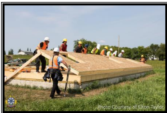
ACC Framing School at Sioux Valley Dakota Nation, students raising an exterior wall.
