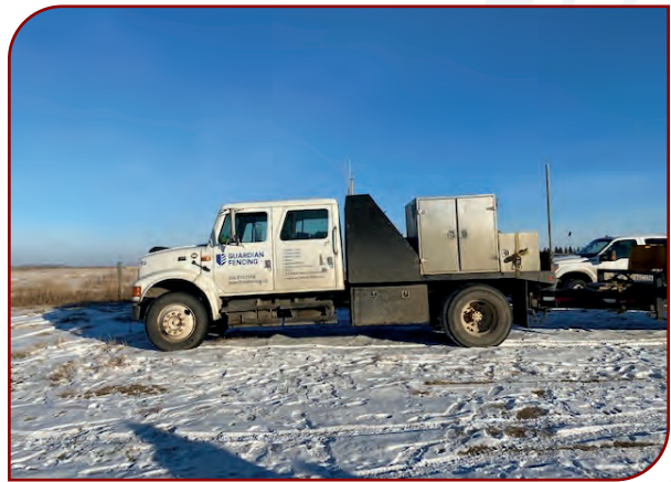
Figure 6. November 24, 2022 – Beginning installation of the new cemetery fence at the Brandon IRS north cemetery site.
